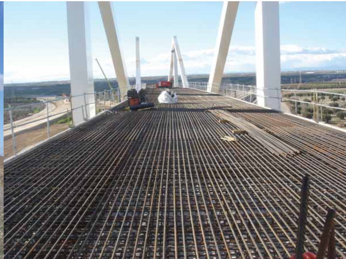
2. Construction supervision of the high speed railway from Valencia to Seville. Detail of bridge over existing railway
